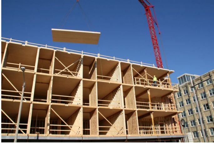
Construction of Timber Lofts apartment building at 331 S. 3 rd St., the first Milwaukee mass timber construction. Credit: Urban Milwaukee.
